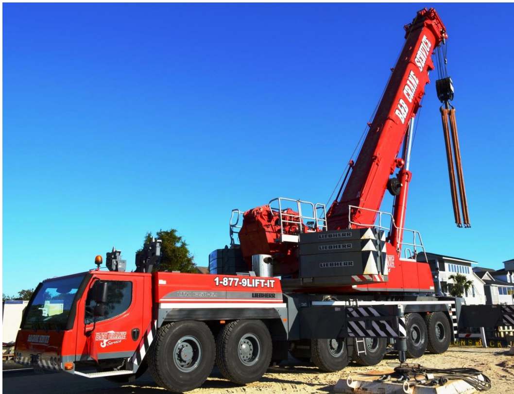
This crane will launch the two dredges and the booster pumps on small barges.
