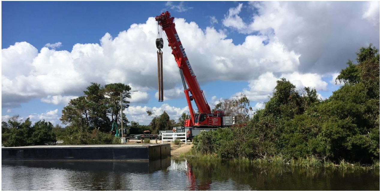
The crane in the background will launch a booster pump on barge shown in foreground. It will also launch the two dredges to be used in the project. (This Photo by Mike Mahaney)
