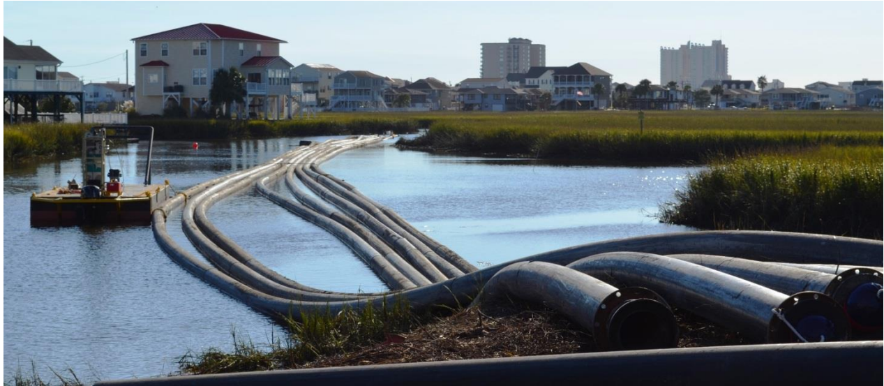
16,000-plus feet of pipeline has been joined together as of October 20. There will be about 20,000-plus feet of pipeline used overall.
